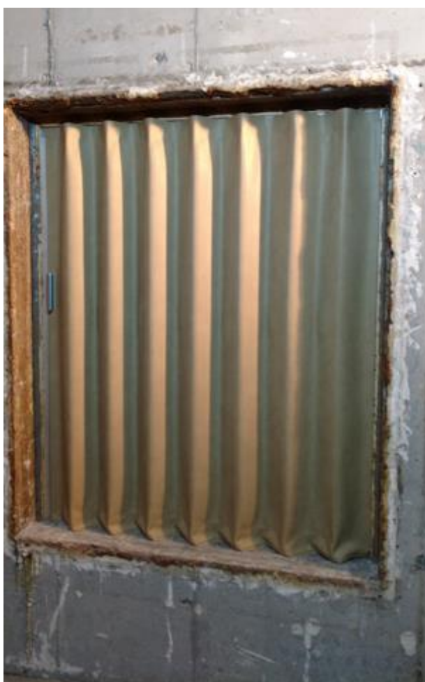
view in Sending Room side
