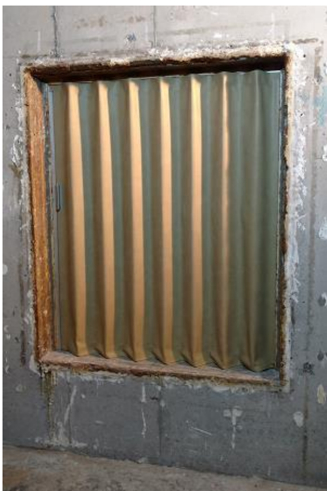
view in Sending Room side
